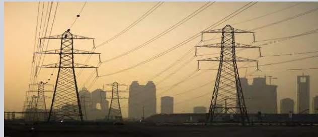
Intelligent energy distribution and transmission
