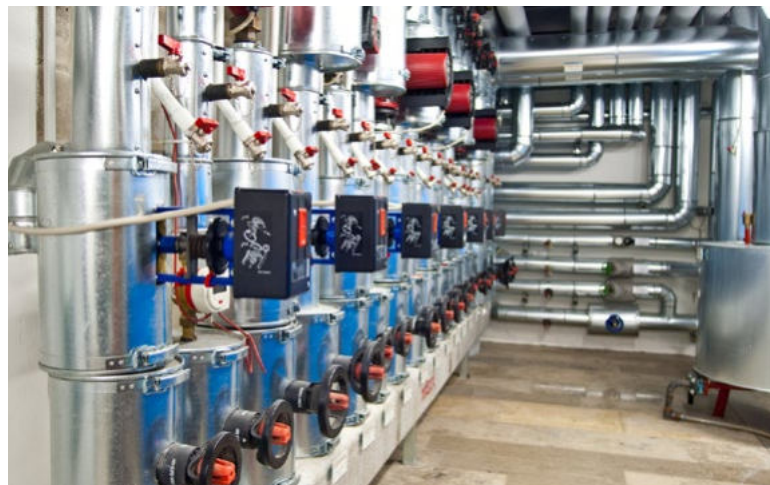
District heating house distributor, photo: stock.adobe.com
