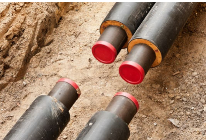
District heating pipes, photo: stock.adobe.com
