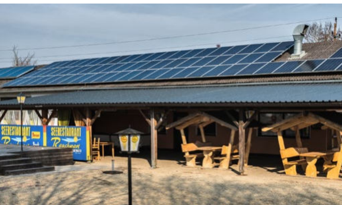
Photovoltaic and charging infrastructure in the innovation laboratory region, Photos: act4.energy
