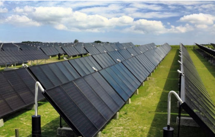
Solar field, photo: stock.adobe.com
