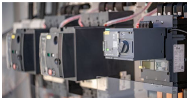
Control units in a smart local substation, photo: AIT/Oleksandr Melnyk
